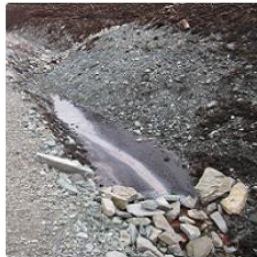
Ditch silted / overgrown or headwall damaged
