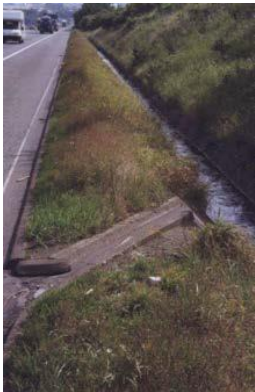
Gully and ditch
